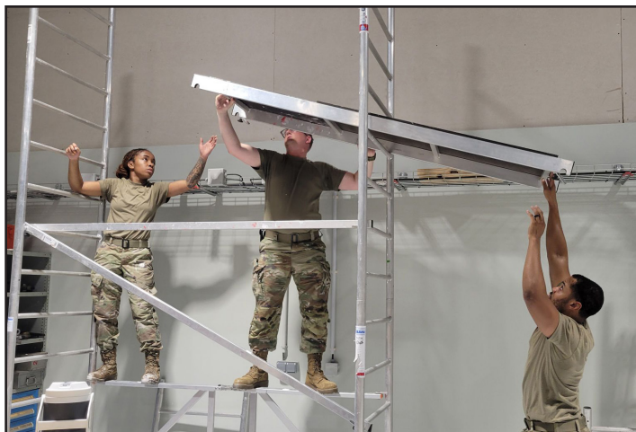
Airmen with the 203rd Rapid Engineer Deployable Heavy Operational Repair Squadron Engineers perform renovation operations July 14-26, 2024, in Azores, Portugal.
